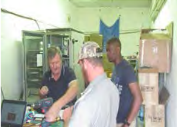
CGS station operators and an official from the PTS inside the Central Recording Facility (CRF) building during the maintenance of the IS47
